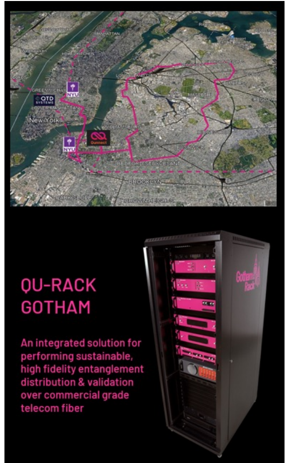
Top Panel – Qunnect’s Gotham Q network spanning Manhattan, Brooklyn and Queens. Lower Panel - QU-RACK GOTHAM enables users to replicate the entanglement distribution protocols performed on the Gotham Q network in NYC.
