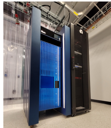
MosaiQ installed in Exaion Data Center
