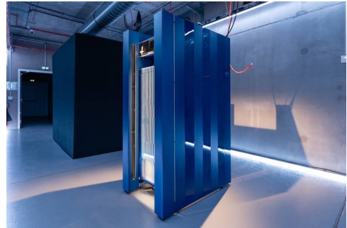
MosaiQ installed in OVHcloud Data Center
